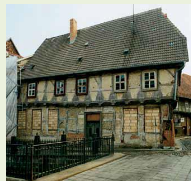
Former merchant's building as part of a courtyard ensemble of urban design significance before...
