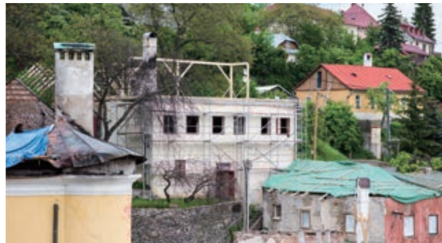
Improvised covering of the damaged houses
