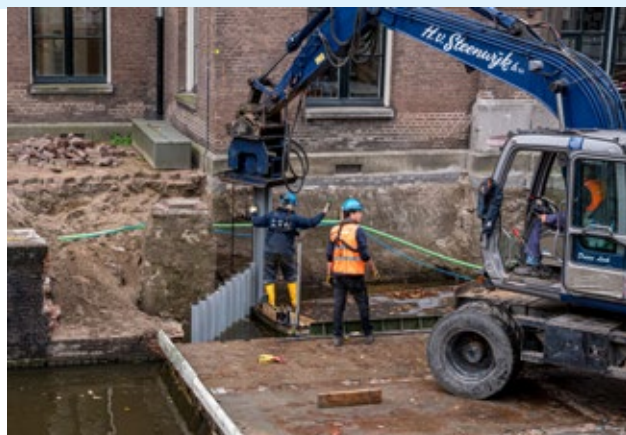
Figure 10: Collapsed quay wall Grimburgwal
